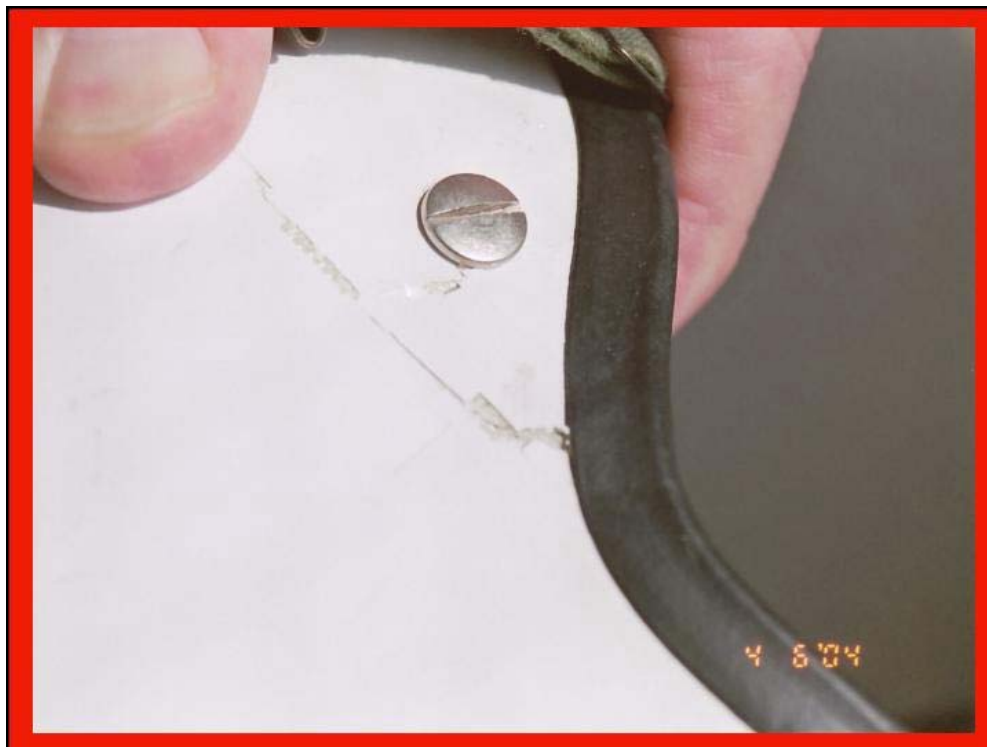
Some cracks are very noticeable.
